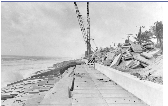
Hurricane Cleo over-washed and damaged highway A1A at the north end of Delray's public beach, 1964. Delray Beach Historical Society Archives
